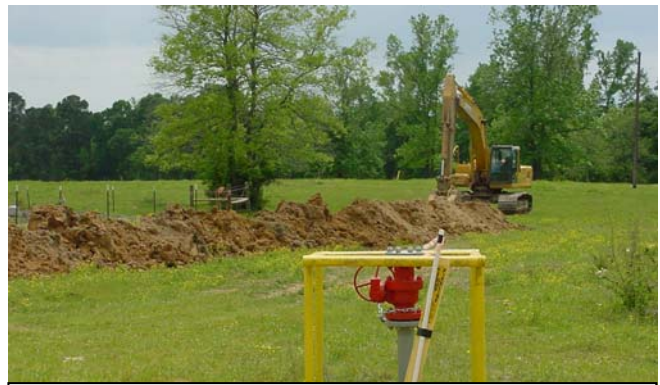
View of 3 rd party riser in foreground, pipeline marker in background
