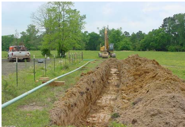
View of the excavation to the point of the line strike
